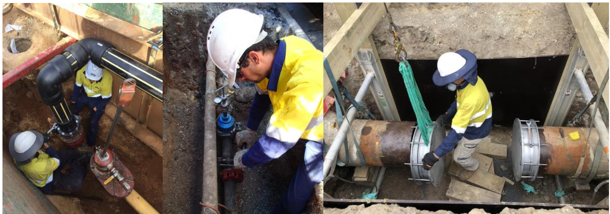
Figure 8.10: (from left) Isolation and bypass on a live steel gas main, South Road, Hindmarsh, April 2017; Mains renewal isolation and cutting activities; Cut and capping low pressure cast iron main, Grote Street, Adelaide CBD, October 2016
